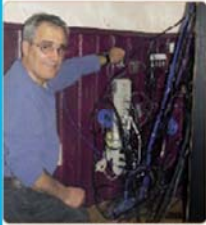
Tony moved his equipment cabinet away from the wall to show us his cabling. He has connected up to six receivers on his antennas. A ADT receiver functions as a central power supply for the LNBs and also acts as the positioner for the actuator motor. All additional receivers are connected as slaves via a splitter or DiSEqC switch.
